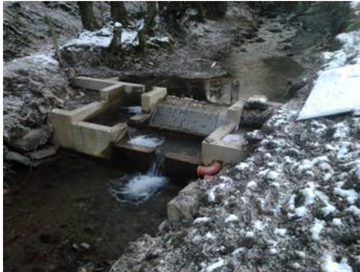
Figure 4 - Intake for 27kW scheme abstracting 50 l/s with integral fish pass
